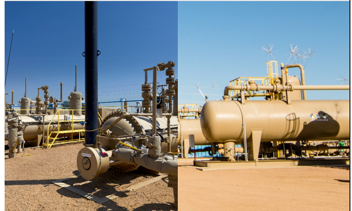
It's important to catch problems with separators early, before they fail, as they are costly to replace.
