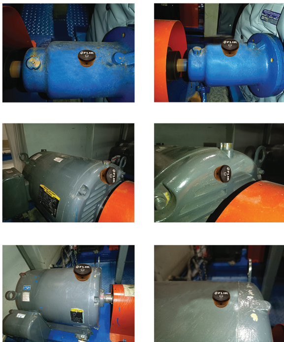
Figure 10.2 Sensors shown mounted on machinery.
