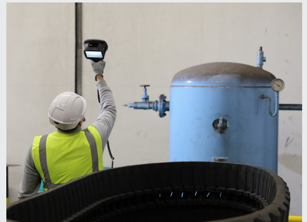
Compressed air systems are used throughout the entire tire-making process and require regular inspections
