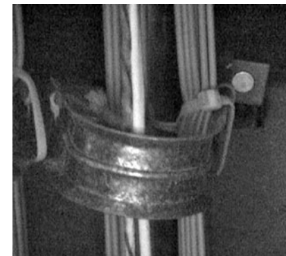
Figure 21 – Example of a common cause of a fiber failure
