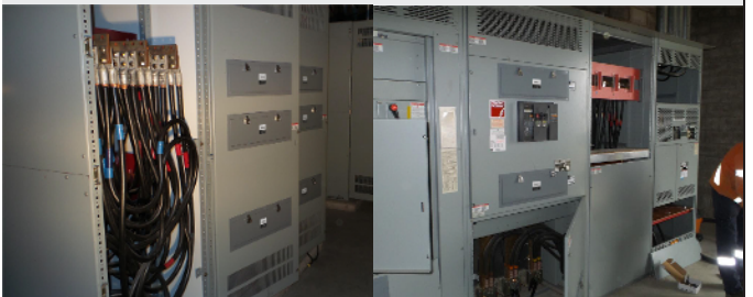
Incoming line connection and main breaker cabinets were also fitted with 24-inch windows
