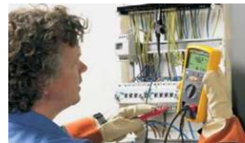
Insulation test at a distribution panel
