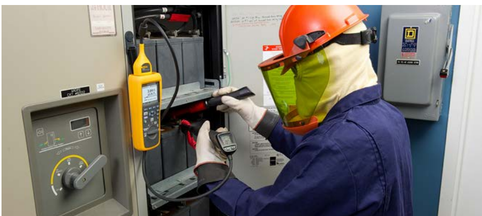
Using the Fluke BT52X to measure impedance, for the quarterly cell/unit internal ohmic value test.
