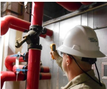
Looking at the water temperature at the inlet to an air handling unit coil.
