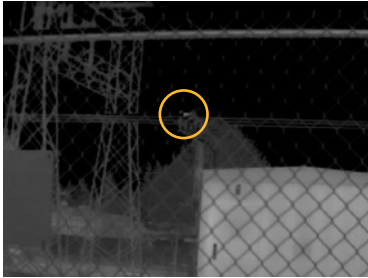
Figure 4. An exterior scan of exterior equipment at a substation with a TiX560 infrared camera and a standard lens captured an anomaly on one of the phase switches.
