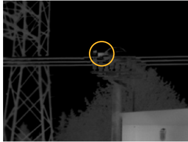
Figure 5. Scanning the same area with a Fluke 2x telephoto lens shows a definite hot spot on the switch.
