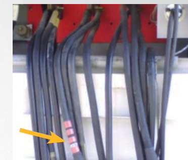
Power Distribution-Full visible
