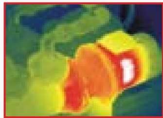
An IR image of a water pump's motor
