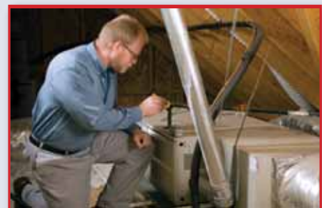
Calibrating HVAC Systems
