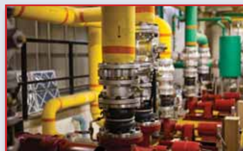
Boiler Room Pump Maintenance
