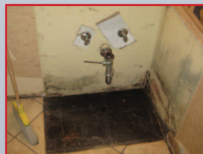
Locate moisture or water damage
