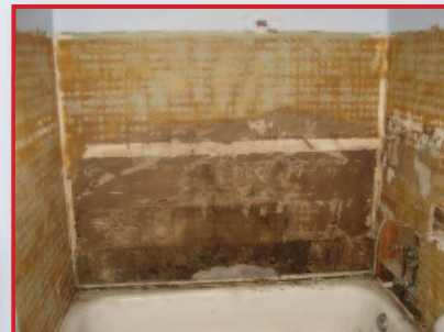
Wet drywall behind removed bathtub tiles
