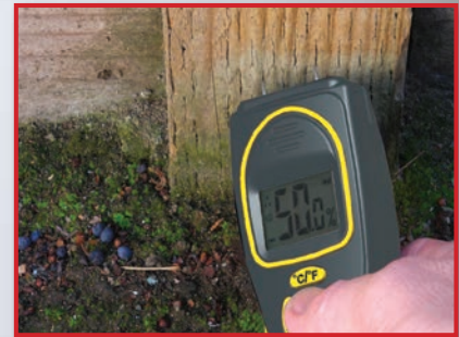
Check wood for dampness or rot
