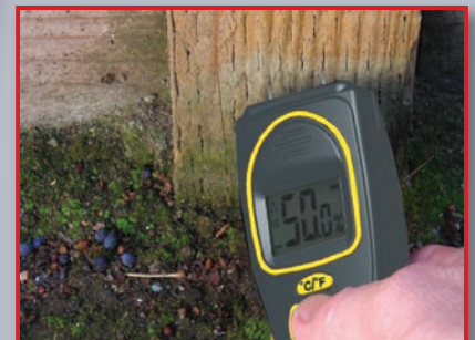
Check wood for dampness or rot
