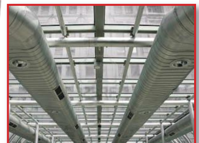
Find blockages or broken registers in A/C ductwork
