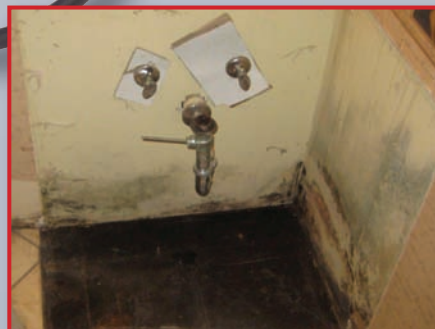
Locate moisture/water damage
