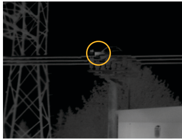
Figure 5. Scanning the same area with a Fluke 2x telephoto lens shows a definite hot spot on the switch.
