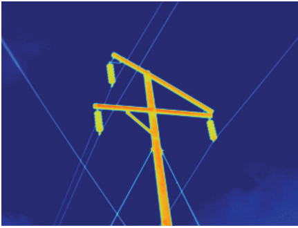
Figure 7: High voltage power pole, captured with a TiX560 camera and standard lens.
