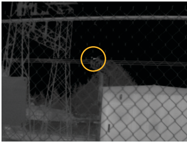
Figure 4. An exterior scan of exterior equipment at a substation with a TiX560 infrared camera and a standard lens captured an anomaly on one of the phase switches.
