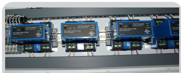
A typical installation of ground fault sensors monitoring several heating circuits used in the semiconductor fabrication process. If a fault to earth is detected, the latching output sensor de-energizes the contactor coil, turning off the offending circuit.
