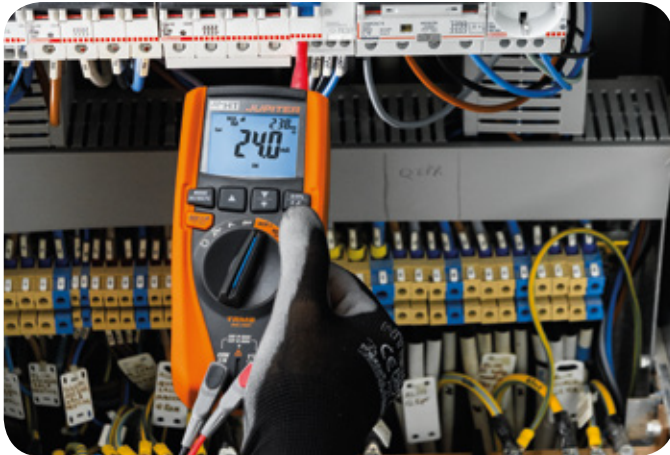
RCD tripping time and current measurement.
