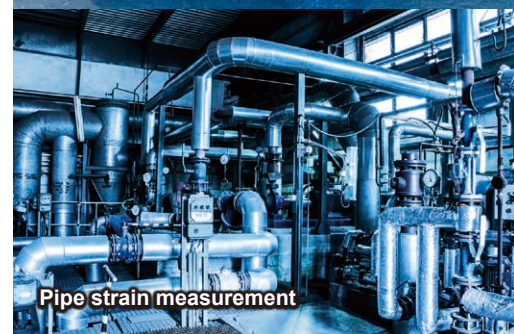
Brake and pipe strain measurement
