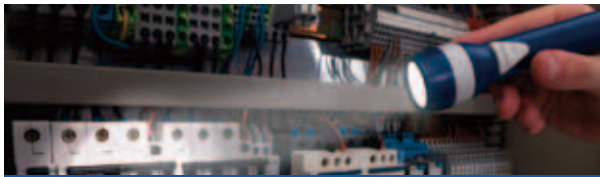
Erroneous circuit-breaker activation
