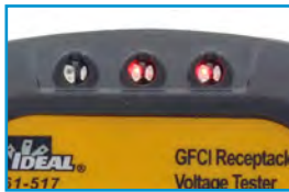
Red Lights Indicate Incorrect Wiring
