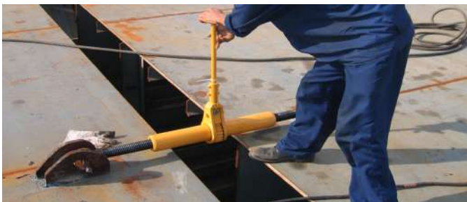
The Loadbinder Jack was used to tie in the sections of this platform. ▼
