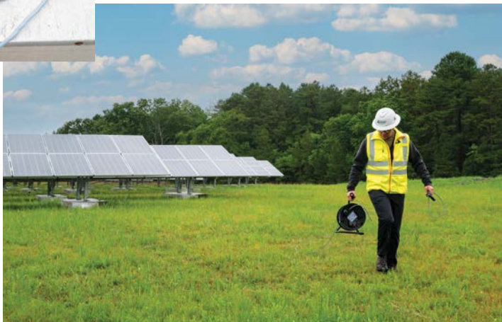
Figure 6-10: In tandem with an extension spool, the DLRO can measure electrical continuity between components up to 100 meters apart.
