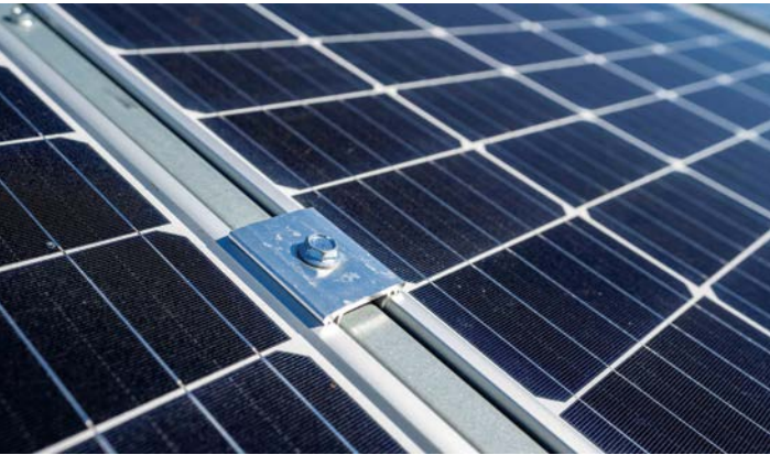
Figure 6-4: Listed PV racking is designed to create an electrical bond between mounting and racking components, and through the anodized layers.
