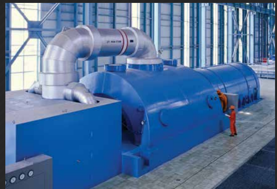
DETECT LEAKS FROM HYDROGEN-COOLED GENERATORS
