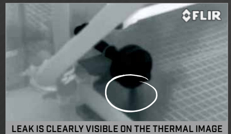
LEAK IS CLEARLY VISIBLE ON THE THERMAL IMAGE
