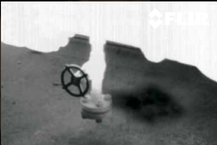
METHANE LEAK AT NATURAL GAS FACILITY SITE
