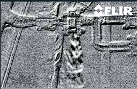
CO 2 LEAK - HSM IMAGE
