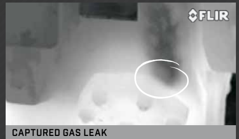
CAPTURED GAS LEAK
