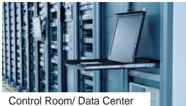
Control Room/ Data Center
