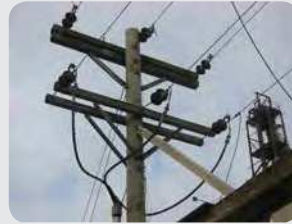
Distribution line faults
