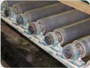
Overheating conveyor bearing
