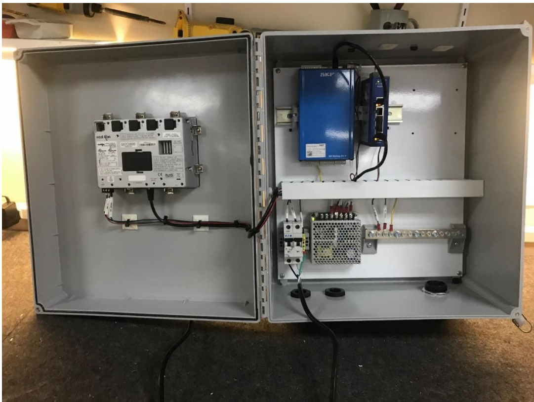
CMCP9000FG-00-HMI09 Inside View
