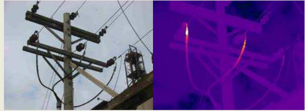
Distribution line faults
