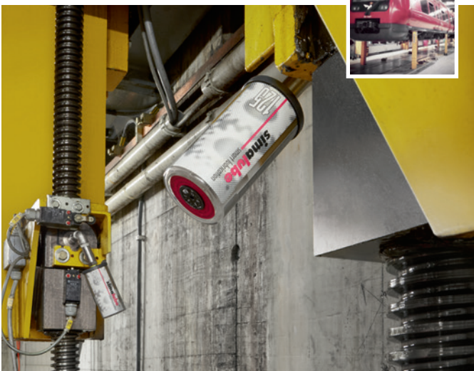
The spindles of a lifting station for railway wagons and locomotives are lubricated with 125 ml simalube over 12 months.
