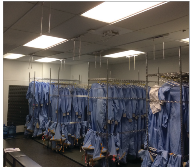
Ceiling Emitters in Gowning Room
