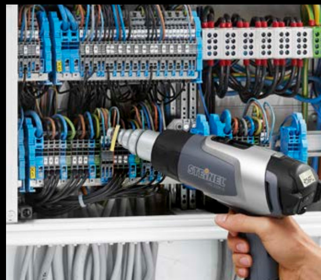
Shrinking cable sleeves in distribution cabinet
