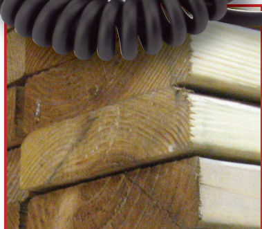
Check wood for dampness or rot
