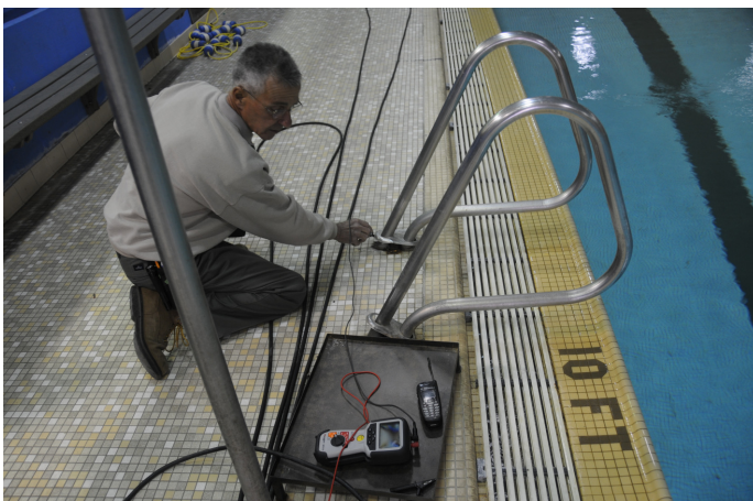
Lou Iaconelli tests a ladder using the Megger MIT420
