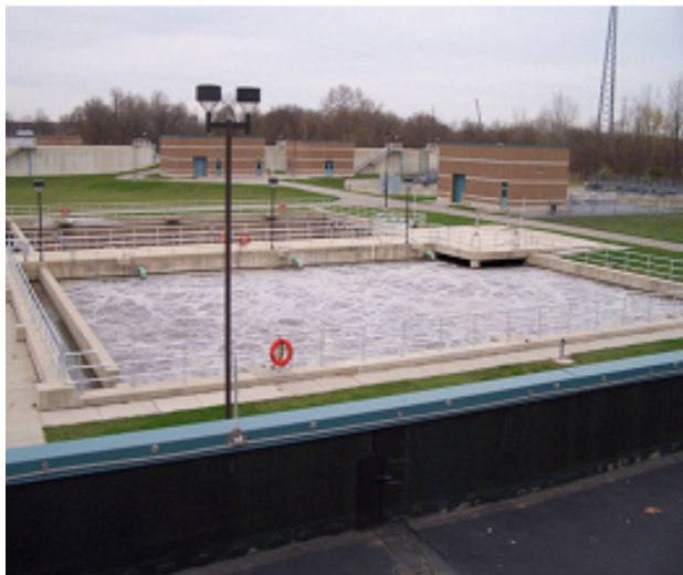
Beaver Creek, Ohio wastewater plant aeration basin.
