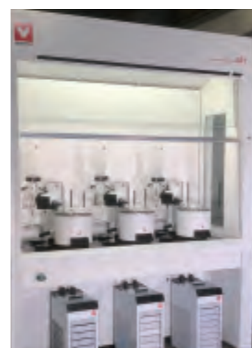
3 vertical type evaporators installed in a fume hood
