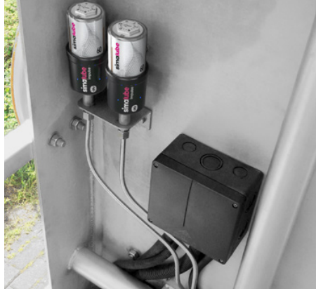
Due to permanently installed lubrication lines on a pool cleaner, two simalube IMPULSE connect are used. They overcome the back pressure and ensure continuous lubrication.
