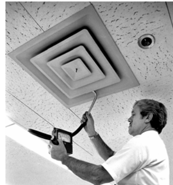
Diffuser measurement using a diffuser probe and deflecting vane anemometer
