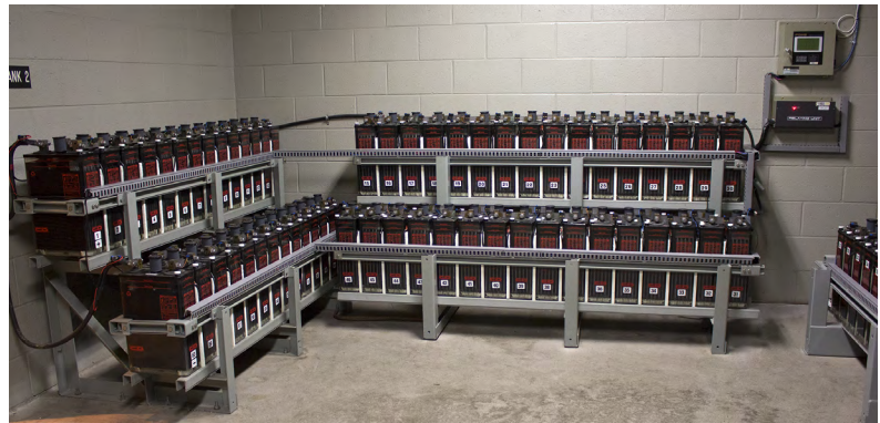
iPQMS Installation on 125VDC Battery System
