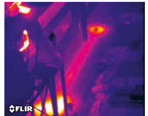
Steam leak underground.
