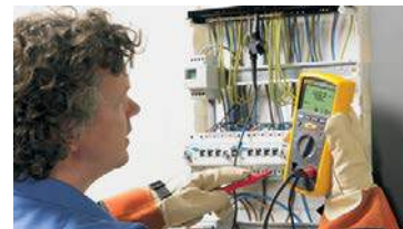
Insulation test at a distribution panel
