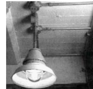
Typical Class 1 Div 1 conduit installation
