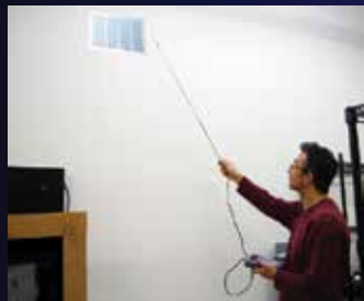
HVAC testing and balancing
