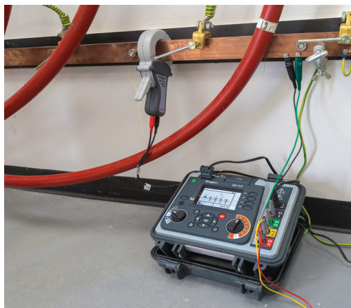
Using ART method with Megger DET2/3 Series to test commercial earth (ground) without disconnecting the system
