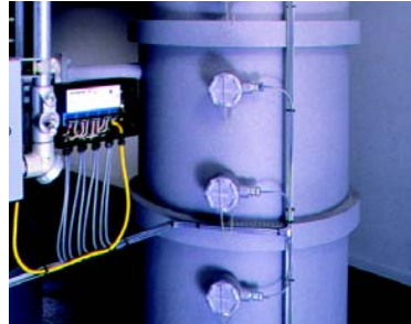
The Rosemount 848T installed.
