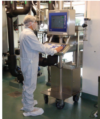
Mobile operator stations provide Novartis with complete flexibility to control its manufacturing process.
