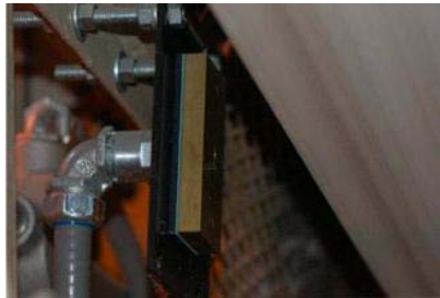
Rub blocks provide an indication when the conveyor is even slightly out of alignment. A conveyor out of alignment can be a potential ignition source.
