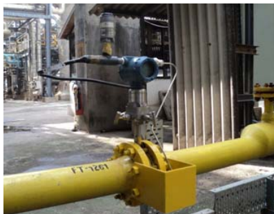
Wireless gas flow measurement with Rosemount 3051SFC and THUM was easily integrated into the plant DCS.
