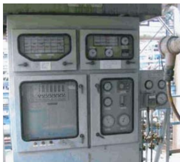
Compressor Control Panel
