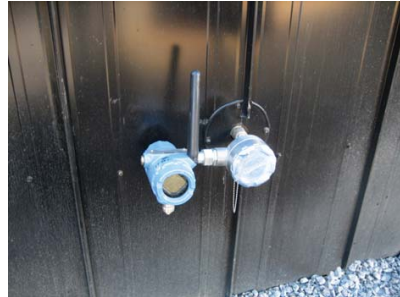
Smart Wireless transmitter on tank.
