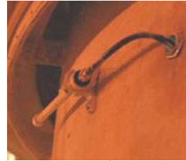
A remote antenna on the center rotating shaft inside the sugar silo allows the wireless instruments to communicate with the Smart Wireless Gateway located outside each silo.
