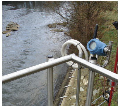
Emerson's Smart Wireless solution monitors river water temperature at the Lenzing Fibers mill.
