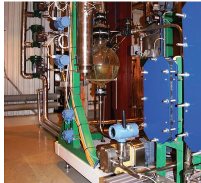
Nine Rosemount wireless pressure transmitters and seven Rosemount wireless temperature transmitters have been installed.
