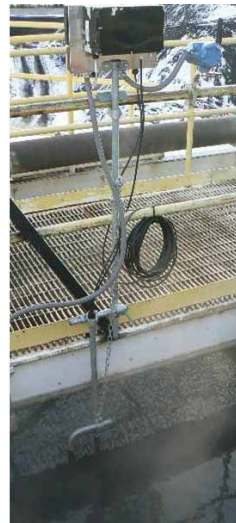
Mobrey MSL600 Sludge Blanket Level Monitor and Rosemount 648 Wireless Temperature Transmitter
