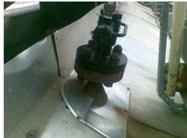
Claus Recovery unit with a Rosemount Application and Industry Solution (AIS) Sapphire Temperature Sensor
