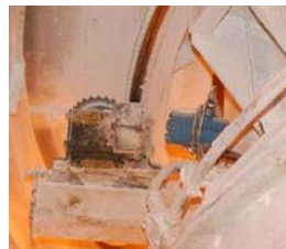
Four 648 (single point) Smart Wireless Temperature Transmitters were placed inside the silos to measure bearing temperatures and motor currents.
