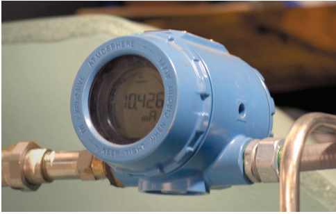
Figure 3.1.3.5b – Remote Mounted Transmitter
