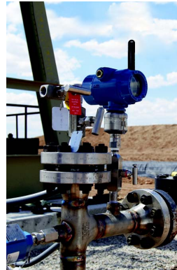
The Rosemount 3051S Wireless Pressure Transmitter Installed
