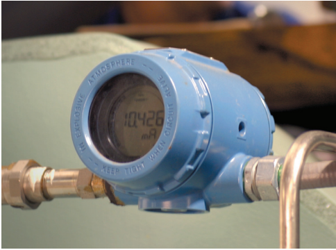
Figure 3.1.3.5b – Remote Mounted Transmitter
