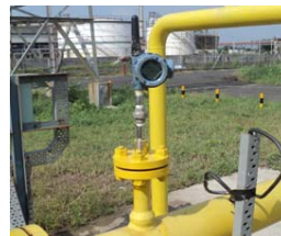
A Rosemount 648 Wireless installed in the Gas Metering Grid.
