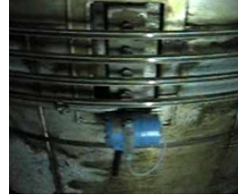
Rotating roaster drum with a Rosemount 648 Wireless Temperature Transmitter
