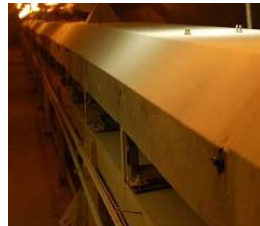
Each of the nine conveyor belts had four bearing temperature measurements and four rub block temperature measurements that were handled by one 848T FOUNDATION™ Fieldbus High Density Temperature Transmitter.
