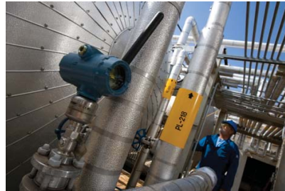
Smart Wireless transmitter installation at BP tank farm.
