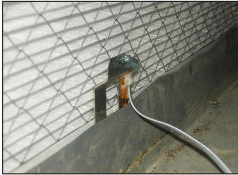
Sensor bracket installed in air handling unit filter tray.
