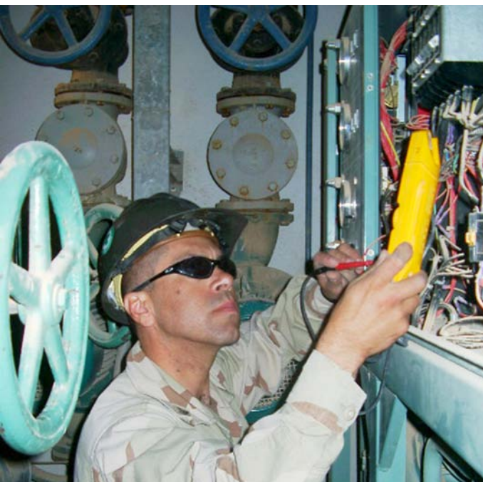
Utilitiesman 2nd Class Pablo Esquivel uses a Fluke Clamp Meter to check voltage on the base theatre chill water plant in Al Asad, Iraq. Esquivel is a member of Naval Mobile Construction Battalion Twenty-Two and deployed to Iraq in support of Operation Iraqi Freedom.
