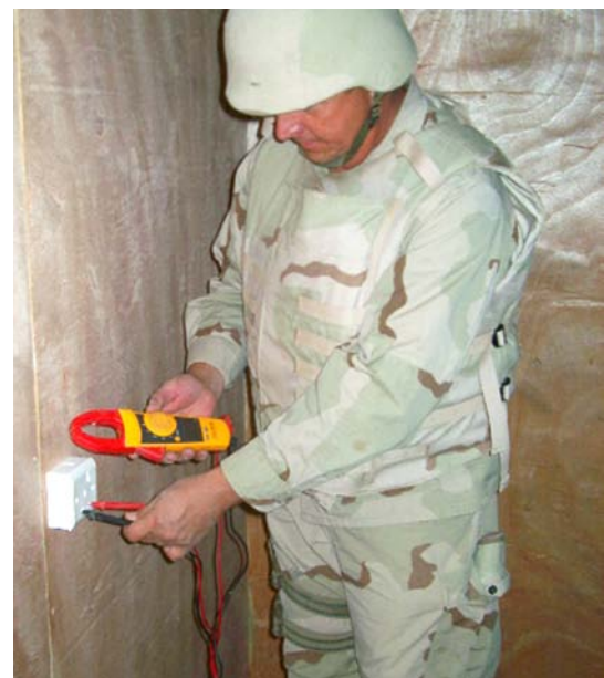
Construction Electrician 2nd Class Grant Wallace uses a Fluke multimeter with an amp clamp to check for proper voltage to an outlet in a Southwest Asia Hut or SWA Hut, a stand-alone wooden multi-purpose structure. The SWA Hut in the photo will be used as a berthing facility for Naval Mobile Construction Battalion Twenty-Two (NMCB 22) members and is located on the NMCB-22 compound in Al Asad Iraq. Wallace is a member of NMCB 22 and deployed to Iraq in support of Operation Iraqi Freedom.
