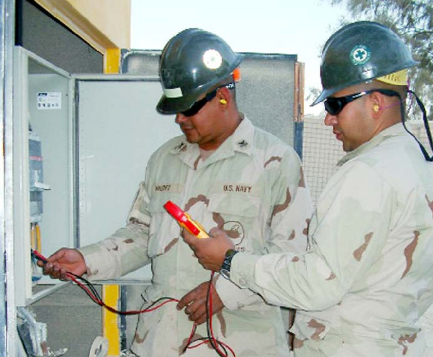
Construction Electrician 2nd Class David Martinez, right and Construction Electrician 1st Class Eddie Valdez use a Fluke Clamp Meter to test the voltage of a generator in order to ensure the correct power needs are supplied to a Marine Corps berthing facility in Al Asad, Iraq. Martinez and Valdez are both members of Naval Mobile Construction Battalion Twenty-Two and are deployed to Iraq in support of Operation Iraqi Freedom.
