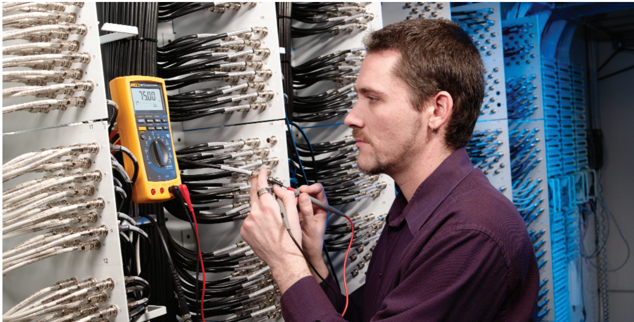
This matrix patch point for coax cable from across the building allows technicians to reconfigure the system on the fly. Here, Grieshaber is performing a quick DC resistance test. Resistance lower than 75 ohms, the standard impedance for video line, could indicate a short, while higher resistance indicates an open circuit or bad termination. With a second technician on the other end of the cable to supply the load, this test can be used to quickly verify cable identity from the lab side.
