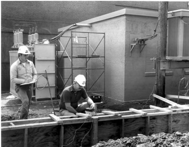
Checking the earth resistance of a ground system at a substation using a Megger ground tester, Cat. No. 250260
