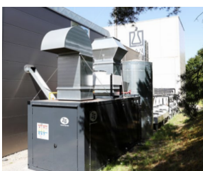
Combined heat and power unit
